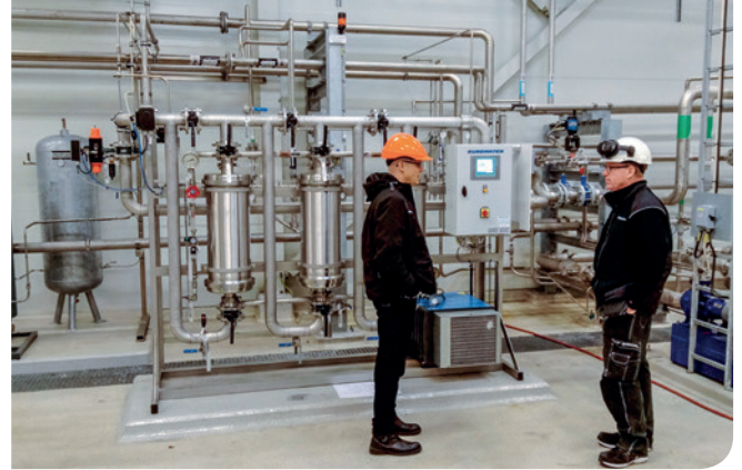
Gothenburg Energy's membrane degasser installation.
