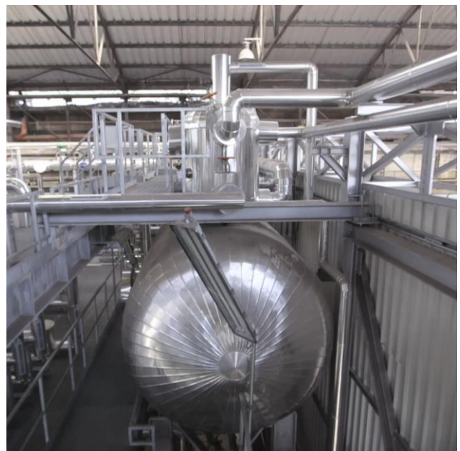
Steam accumulator and steam pipes. Source: ORI MARTIN
