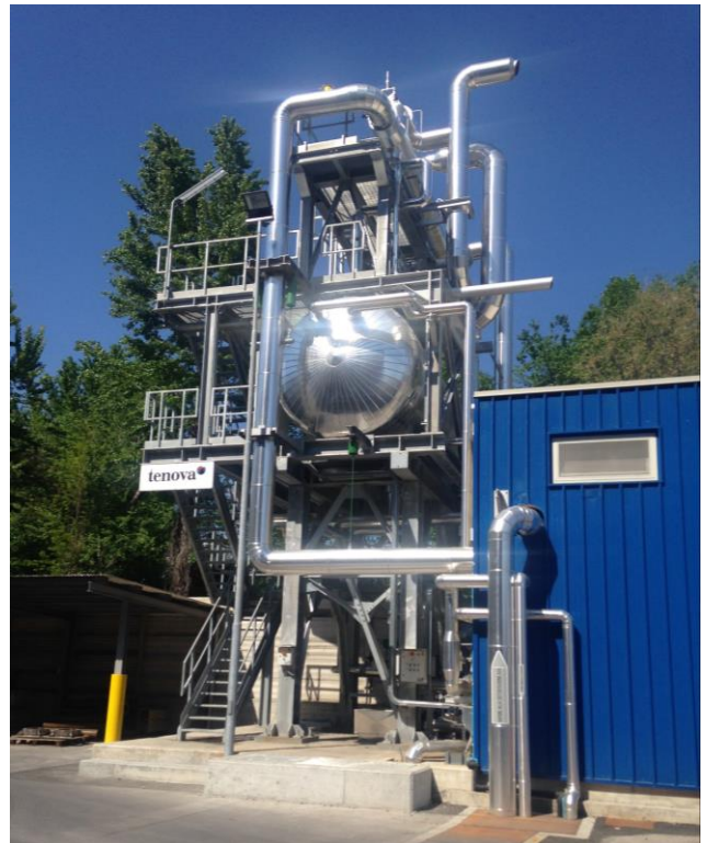
Heat substation for heat delivery to the district heating network operated by A2A. Source: ORI MARTIN
