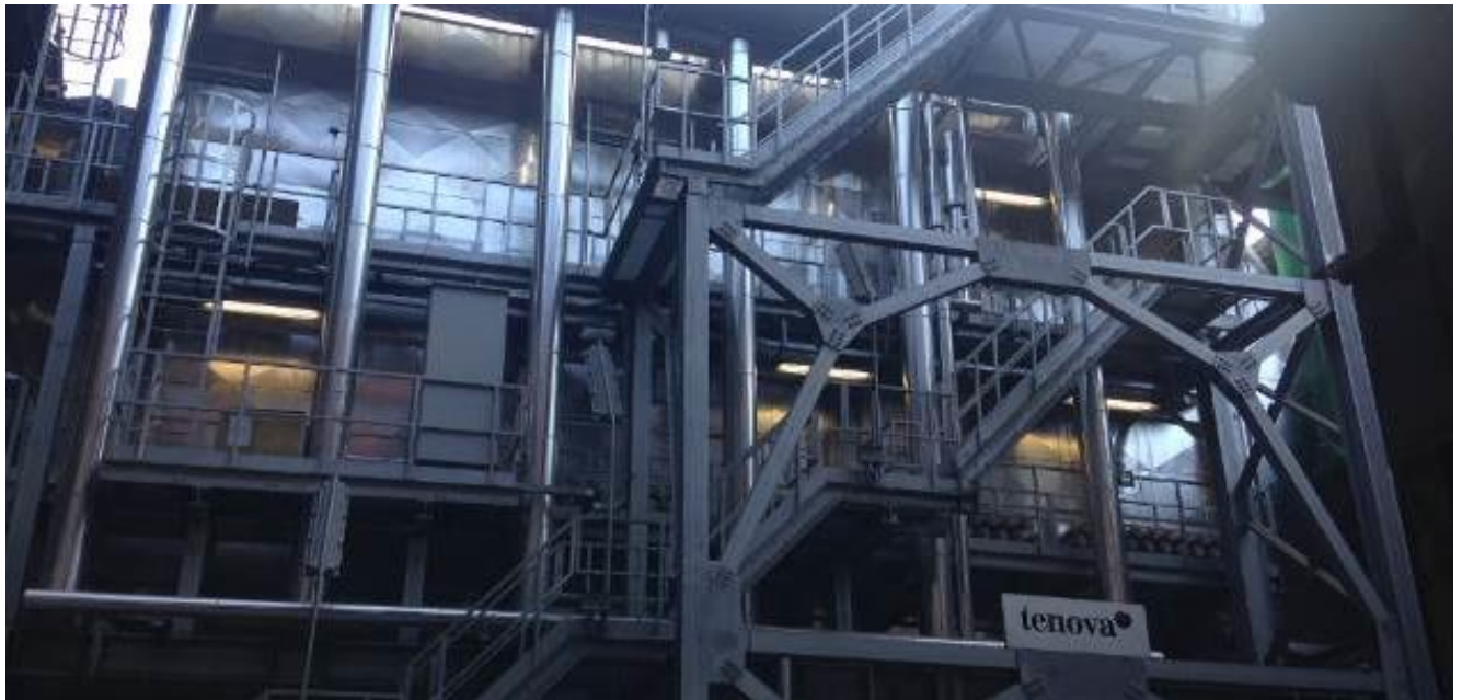
Waste Heat Recovery Unit. Source: ORI MARTIN
