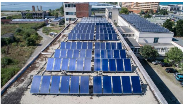
Figure 42: Solar heating installation including 700m 2 solar collectors for Pomorie Hospital – in operation. Source IZEB
